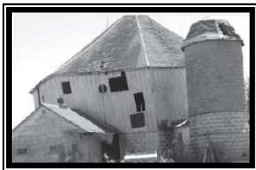
Leaning Silo of Drywood
